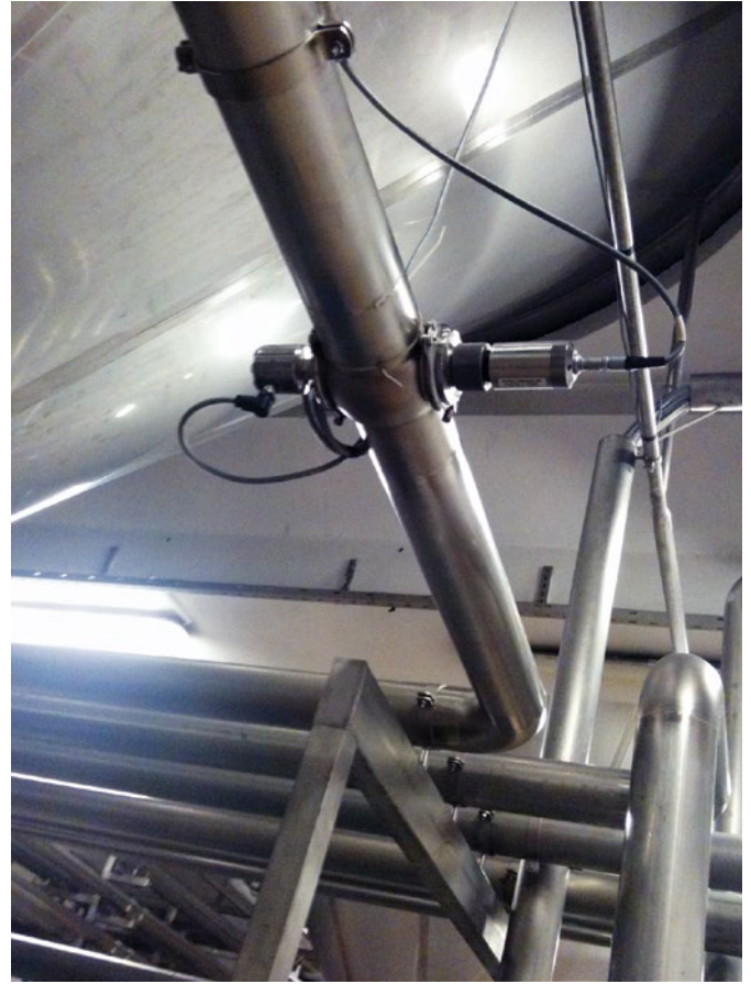
Abb. 3. Hach M1100-H LDO-Sensor – typische Installation
